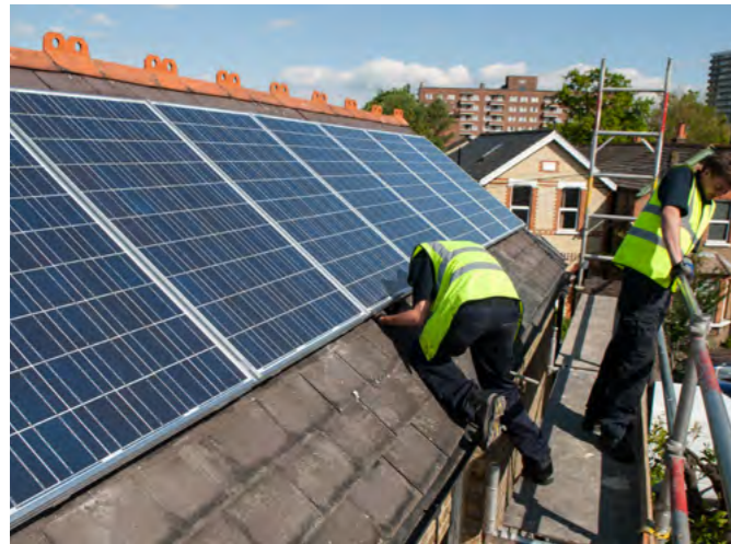
Figure 11 Solar Panel installations
