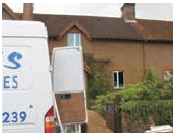
Inappropriate plastic windows being installed in an Aldbury cottage
