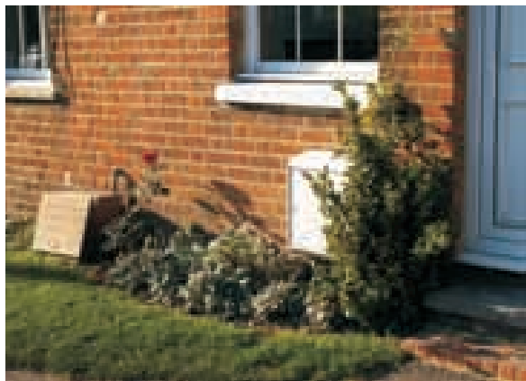
Meter boxes should be handled sensitively: exposed plastic boxes can be concealed in more appropriate timber enclosures
